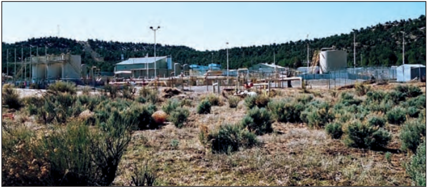
Compressor stations like this one off the Rosa Road in the San Juan Basin run 24 hours a day, seven days a week, filling the air with noise and diesel exhaust. (Joel Gay)
